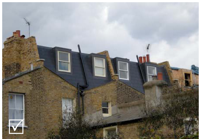
Fig 5.36: Acceptable - Butterfly form retained with slope of mansard running down to meet the existing eaves (please note that proposals should not include drainpipes)
