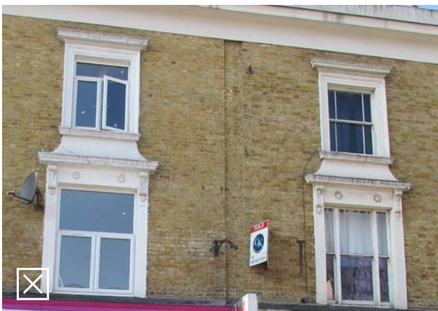
Fig 6.1: The replacement of traditional style windows on heritage properties with modern UPVC windows can be hugely detrimental to the properties character
